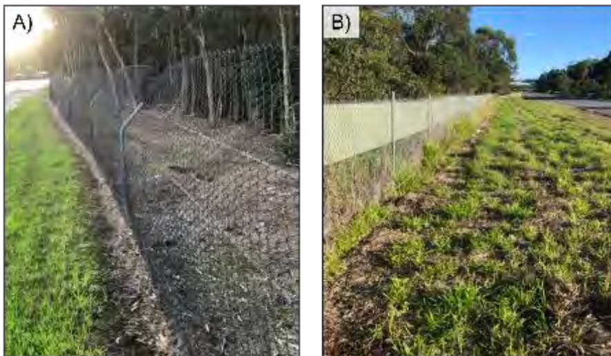
Figure B.6.7 A) 'Floppy top' wildlife fencing and B) 1.5 m high chain mesh fencing with metal flashing (Source: Sandpiper Ecological)
