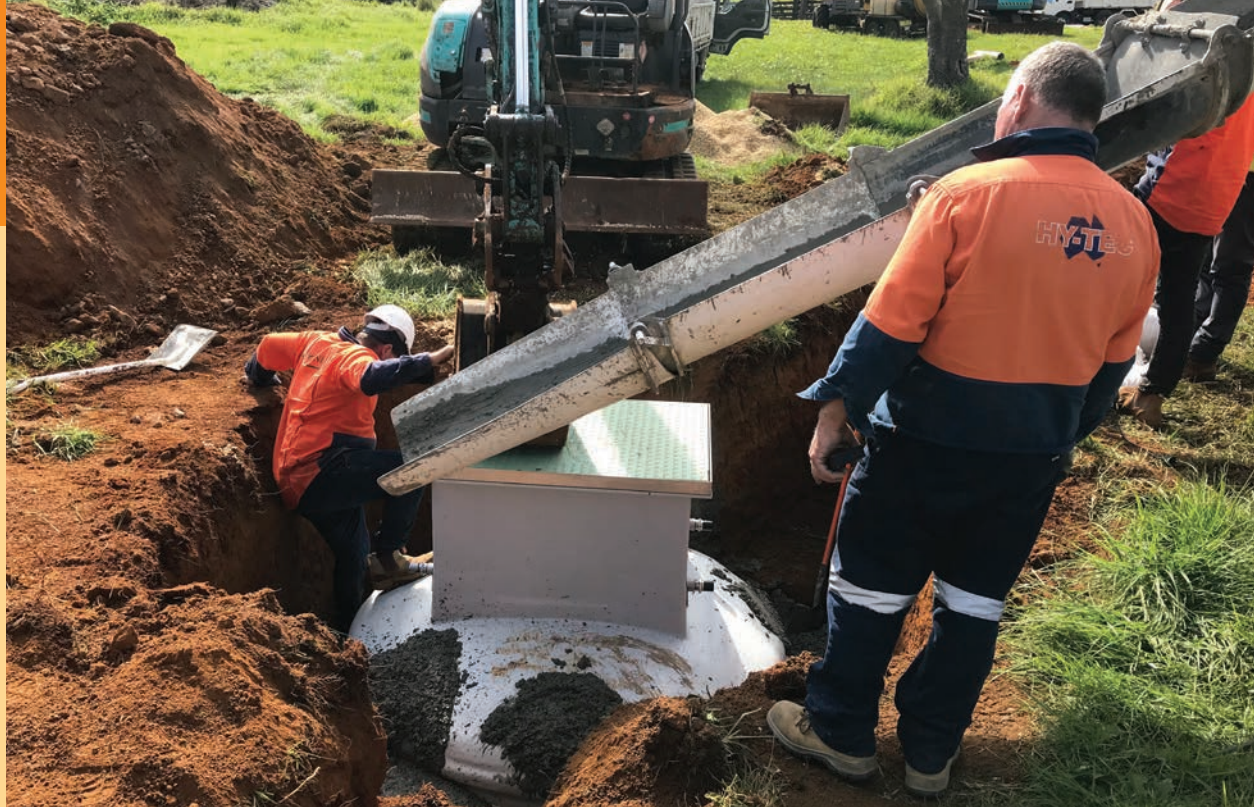
Comboyne sewerage system
